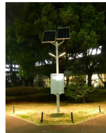
Autonomous street lighting at night
