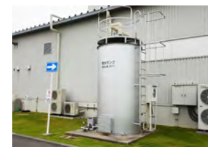
Rainwater storage tanks (Okazaki Plant)
