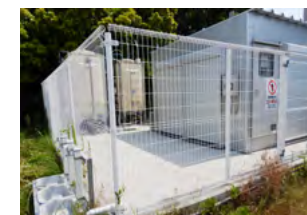
Groundwater membrane filtration equipment (Okazaki Plant)
