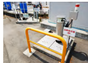
Surface oil detector (Okazaki Plant)
